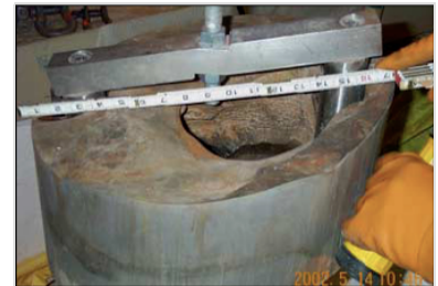
Erosion of the 6-inch-thick (150 mm) carbon steel reactor head, caused by a persistent leak of borated water
